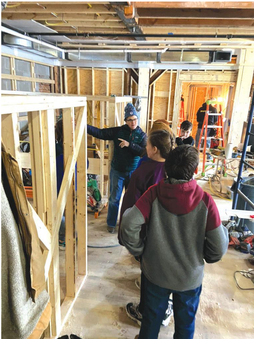
FIFTH- AND SIXTH-GRADE students from Neshobe toured the ongoing renovation of the Brandon Free Public Library as part of their field trip to Naylor & Breen, which is supervising the work.
